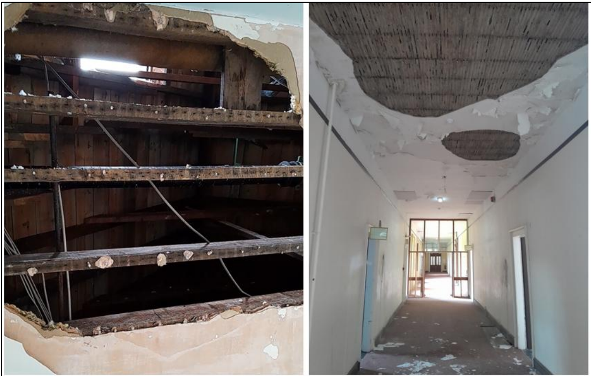
Figure 8.31: Images showing the level of disrepair of the ceilings and attic floor in Tabor House. Daylight can be seen through a skylight in the roof in the left-hand image (Source: DNV).
