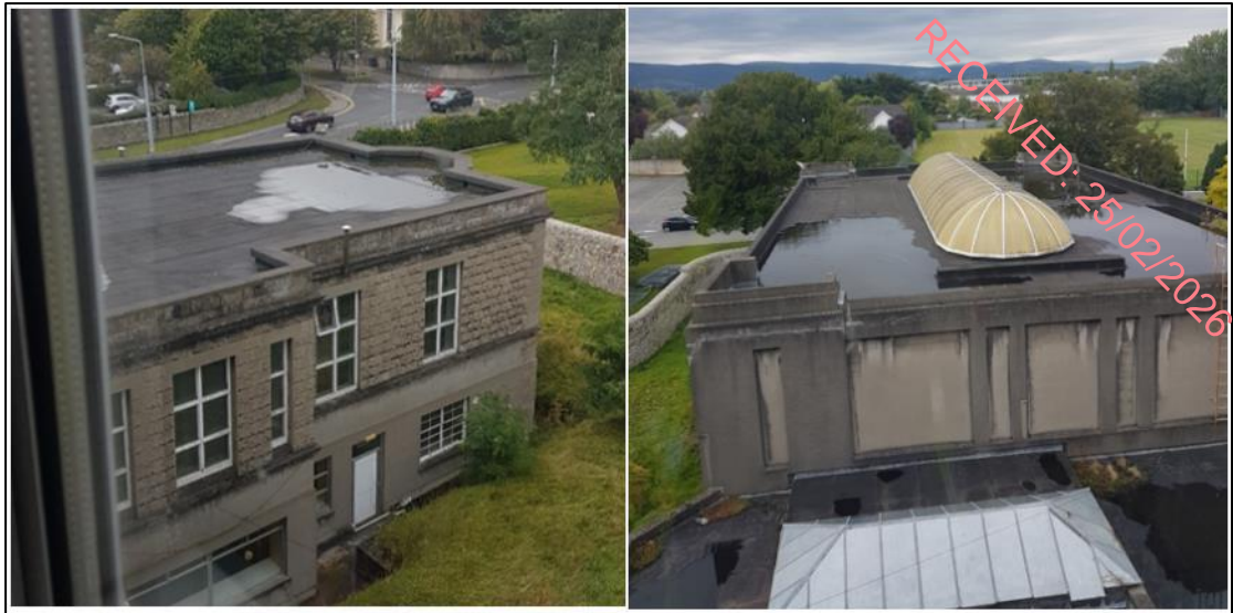
Figure 8.37: Views of the roofs of the Finlay Wing (left image) and the Archive (right image) from Milltown Park House (Source: DNV).
