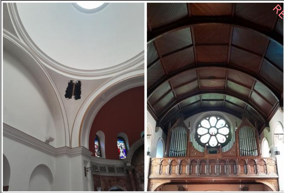
Figure 8.33: Images of the Chapel ceiling showing intact internal structure other than one piece of damage (Source: DNV).
