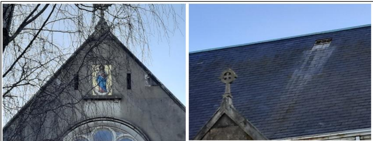
Figure 8.34: Examples of PRFs (vents) on The Chapel's eastern gable end and roof (Source: DNV).
